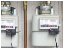
Impulse counter "Elster" to diaphragm gas meter
